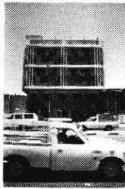
Fig.45 Exposed steel bars and concrete columns. Baghdad, 1960-70s
