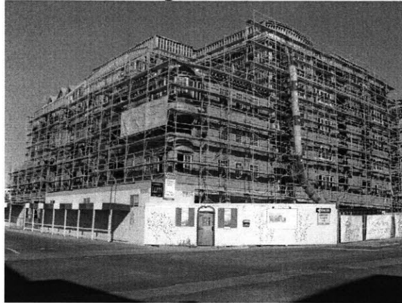
Additional residential buildings are under construction all over the Little Italy station area.
