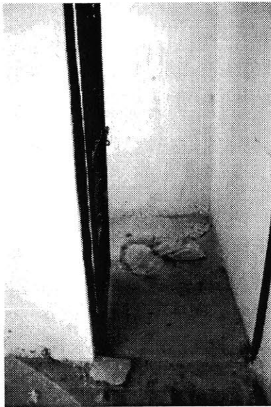
Fig.24 The lavatory is not used because it is not connected to a sewage system
