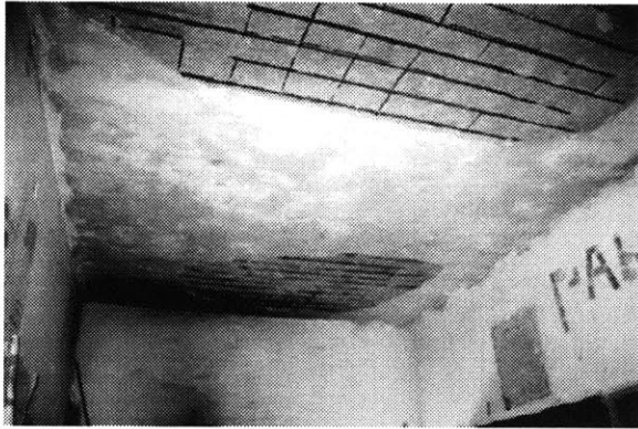
Fig.3 Crumbling ceiling in a government school
