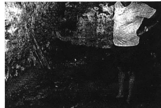
Example of basement conditions of a home in the Mill Creek Neighborhood. Photo: web.mit.edu/wplp/home.htm
