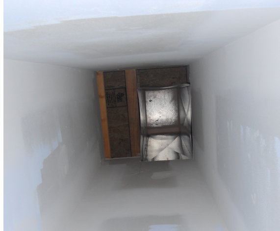
Figure 4.9. The laundry chute goes through the rafters without a barrier.
