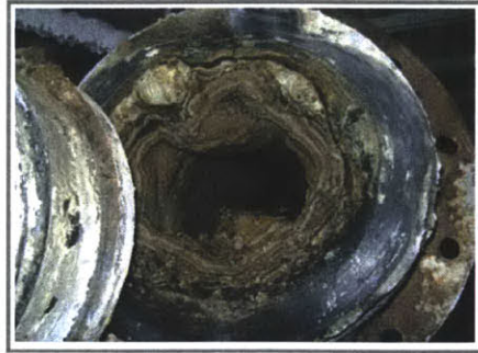
Figure 4: Opened Water Pipe
