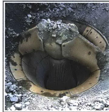
Figure 11: Gyratory Crusher in operation.
