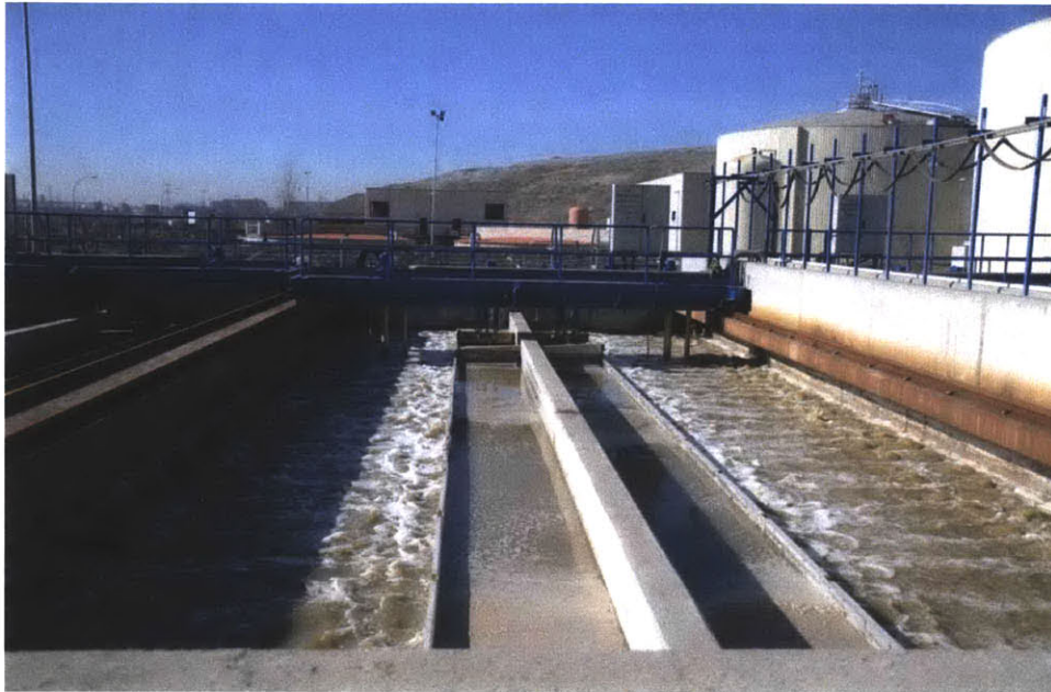
Figure 2.11 Aerated Grit Chamber
