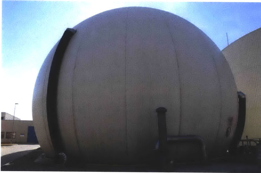
Figure 2.14 Gasholder for Biogas Produced from Sludge Digesters
