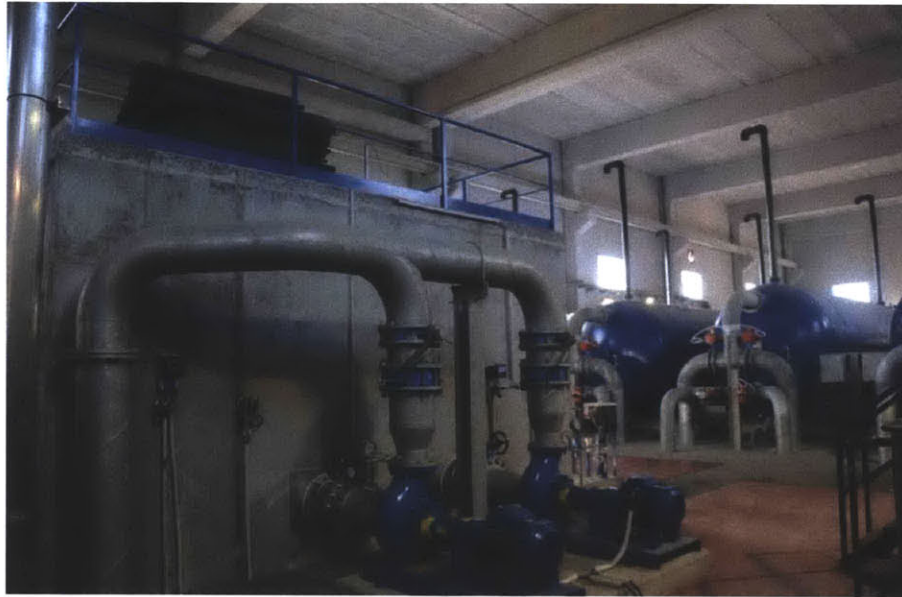
Figure 2.13 Tertiary Treatment: Filtration Tanks and UV Disinfection
