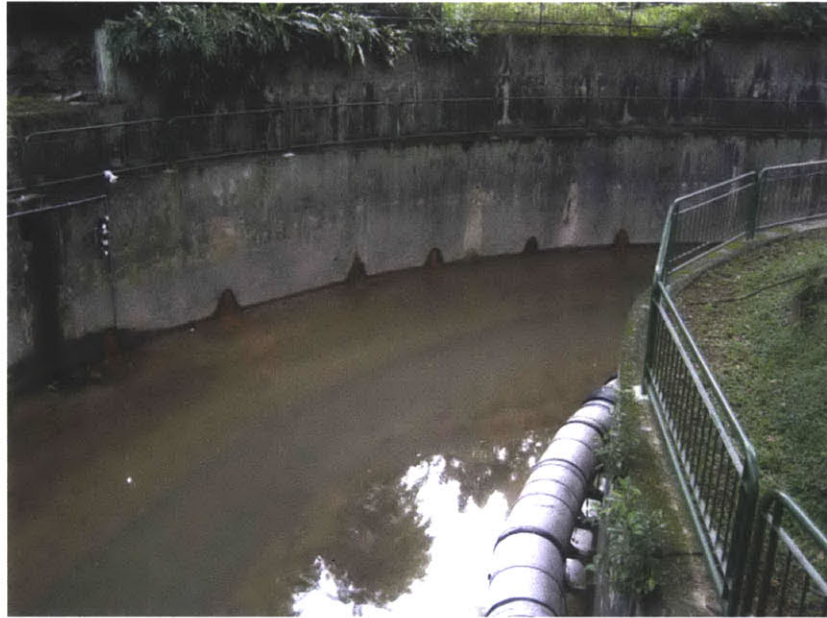
Figure 16 – Pressure release nodes in a large drain (Photo: Laurie Kelldorfer)
