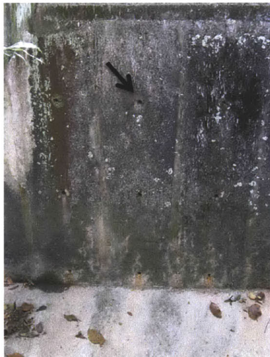
Figure 15 – Close-up of pressure release nodes on the sides of drains (one of several nodes is highlighted by an arrow) (Photo: Laurie Kelldorfer)
