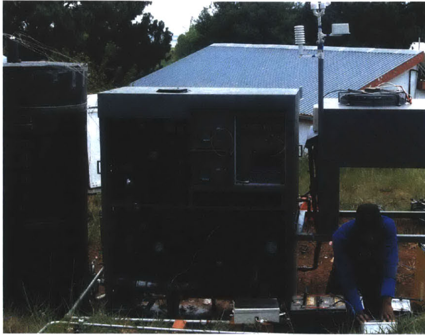
Figure 4-15: 3kW e ORC built in Lesotho in partnership with ATS and STG.
