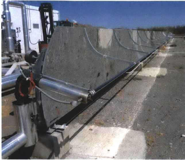
Figure 4-18: NEP solar collector field at Plataforma Solar de Almería, Spain
