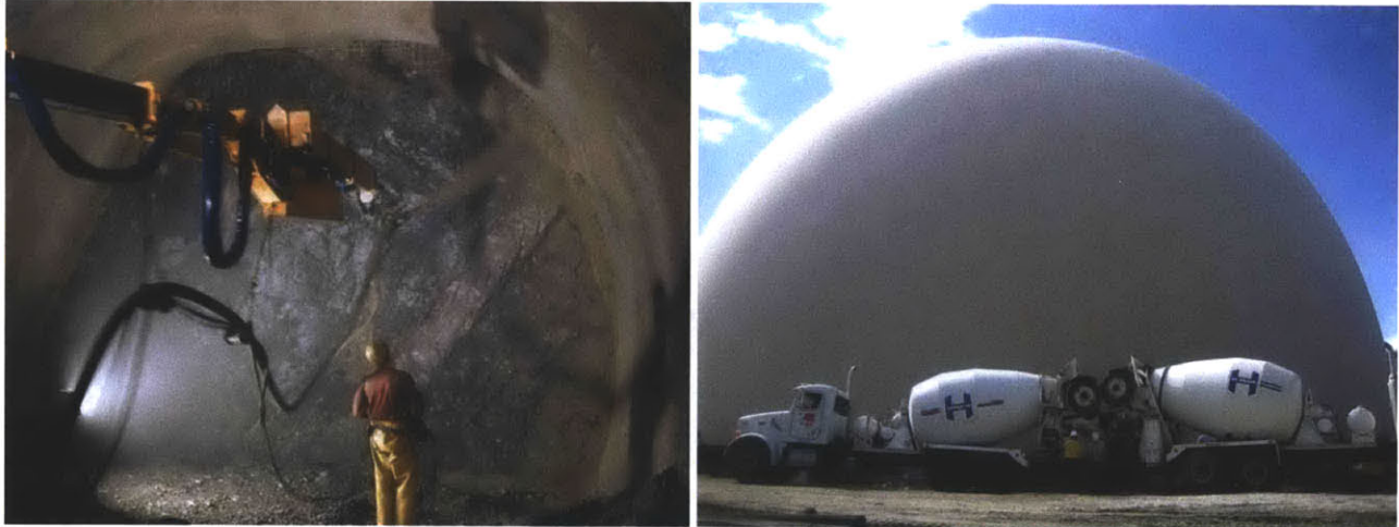
Figure 30 Automatically executed shotcrete (on the left Source: http://www.multicretesystems.com/shotcrete ) and shotcrete dome (on the right source: http://www.reedpumps.com/concretedomes.htm )
