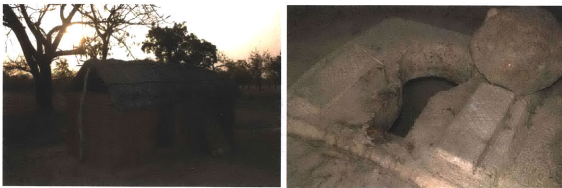
Figure 38: One of the latrines in the Suburi Village (left) and the DA-provided concrete slab with cover inside (right)
