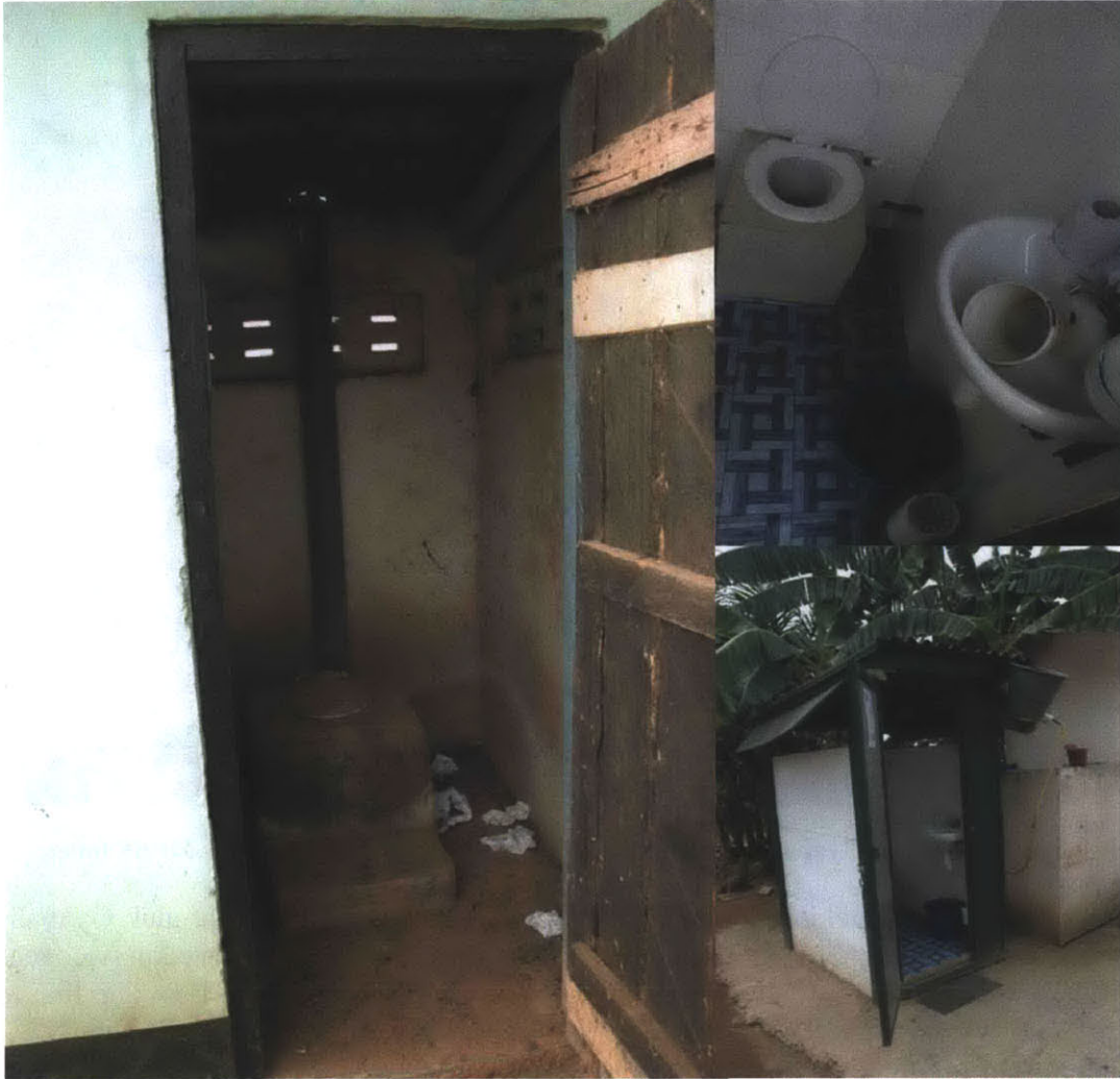
Figure 44: The old VIP latrine still being used by Samuel's father (left) and the new MFBF toilet facility (right-below) with an enlarged view of the sink and toilet (right-above)
