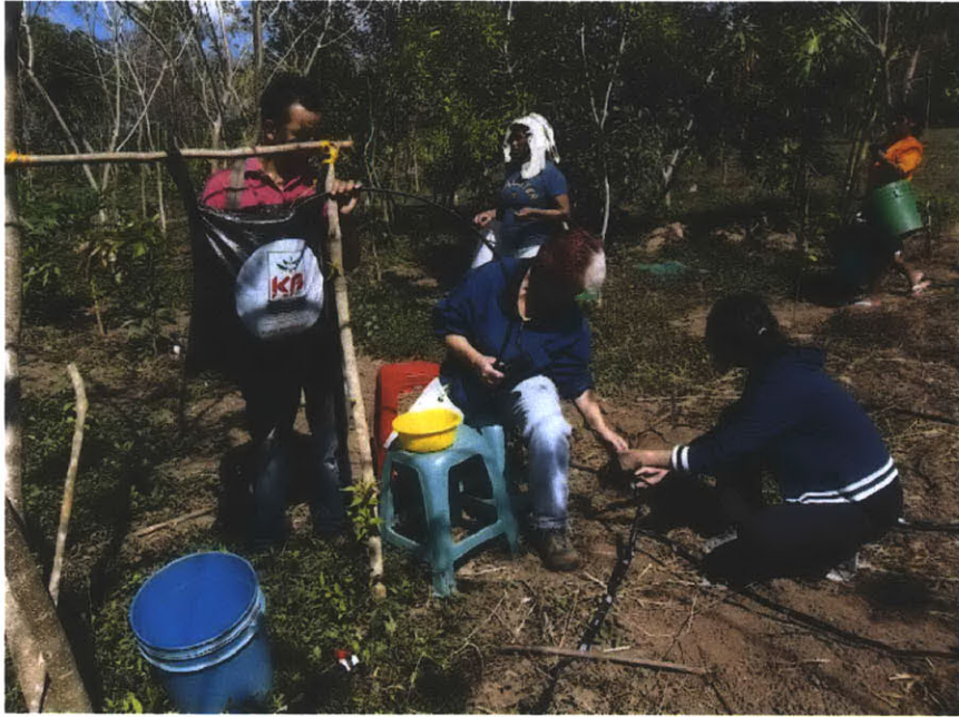
Figure 5.4: Pumping the system to start the flow rate. Photo: Susan Kinne (2012)
