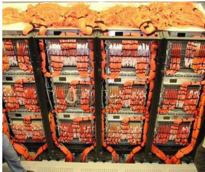
Figure 1- 4: Central switch racks, Barcelona Super Computing Center.
