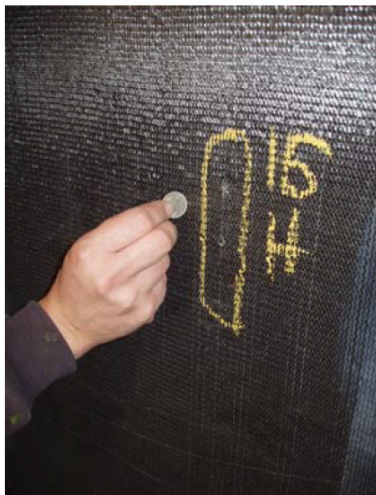
(c) Two found air voids
