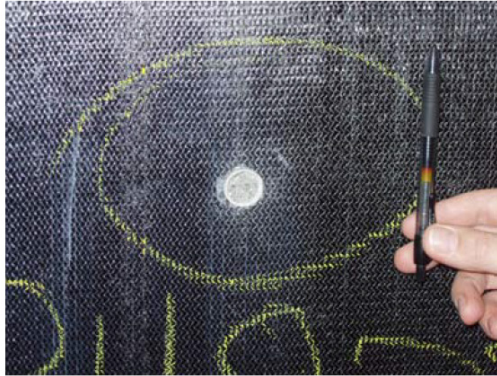
(a) Found air void defect with the removal of GFRP sheet
