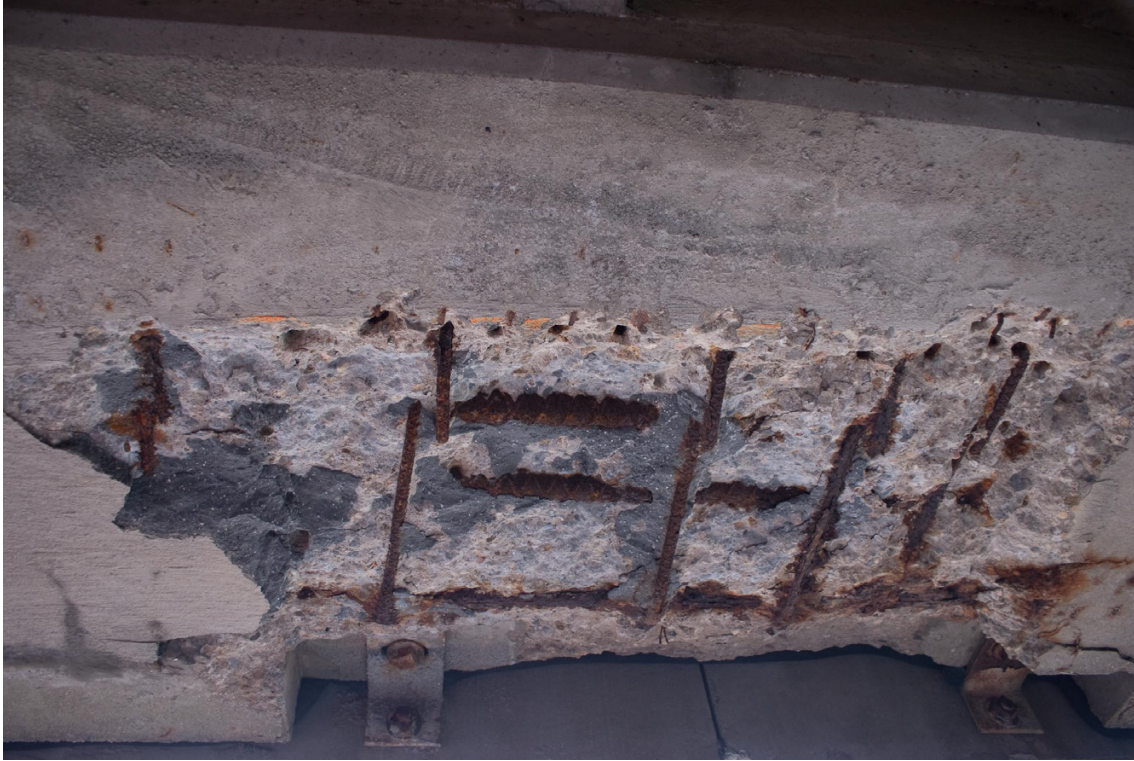
Figure 1-2: Corroded rebar and concrete spall, MIT Campus, West Garage
