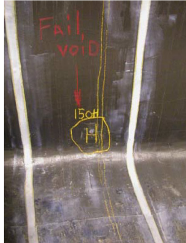
(b) Air void found near the corner
