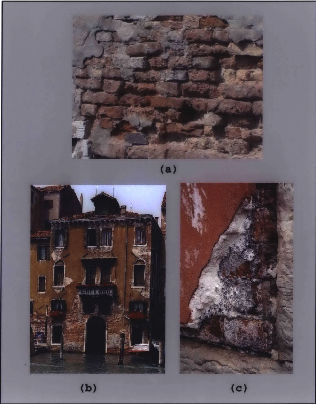
Figure 1-1: Examples of weathering effects on Venetian building facades.
