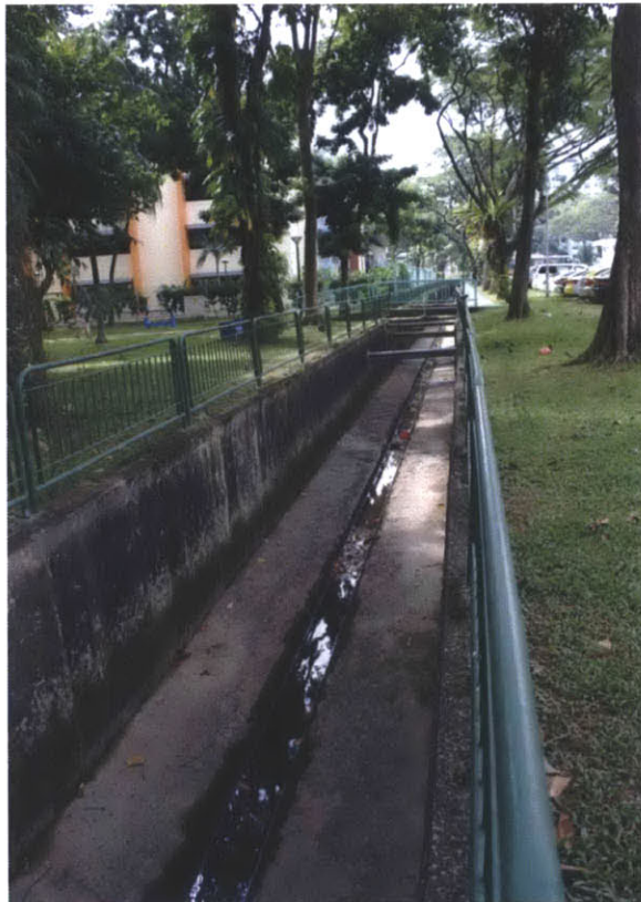
Figure 11. The main drain at Lorong 8 Toa Payoh, where C1 and C2 are located.
