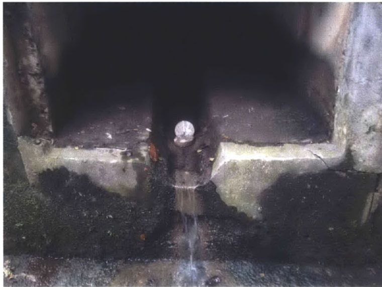
Figure 9. Concrete coupon C1 in the tributary at Lorong 8 Toa Payoh with a vertical concrete coupon upstream to block debris.
