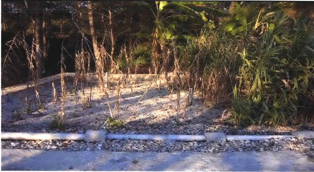
Figure 5.8: Horizontal Flow Bed at SKM Hospital
