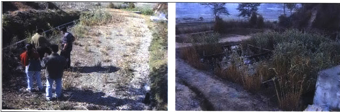
Figure 5.3: Horizontal Flow Bed (Left) and Vertical Flow Bed (Right) at Dhulikhel Hospital
