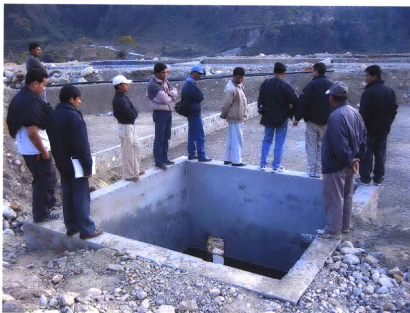
Figure 5.18: Intermitted Feeding Tank for Horizontal Bed.
