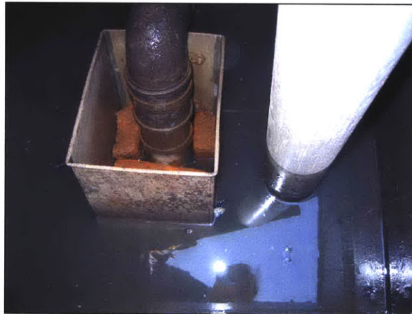
Figure 5.10: Hydro-mechanic Feeding Tank
