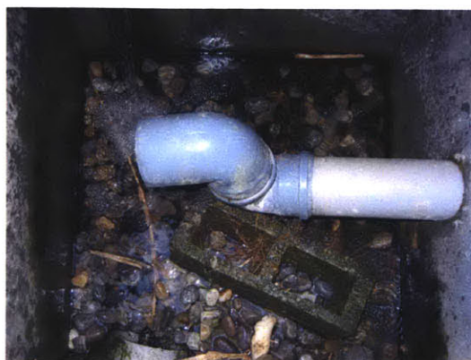
Figure 5.12: Effluent of the Constructed Wetland System
