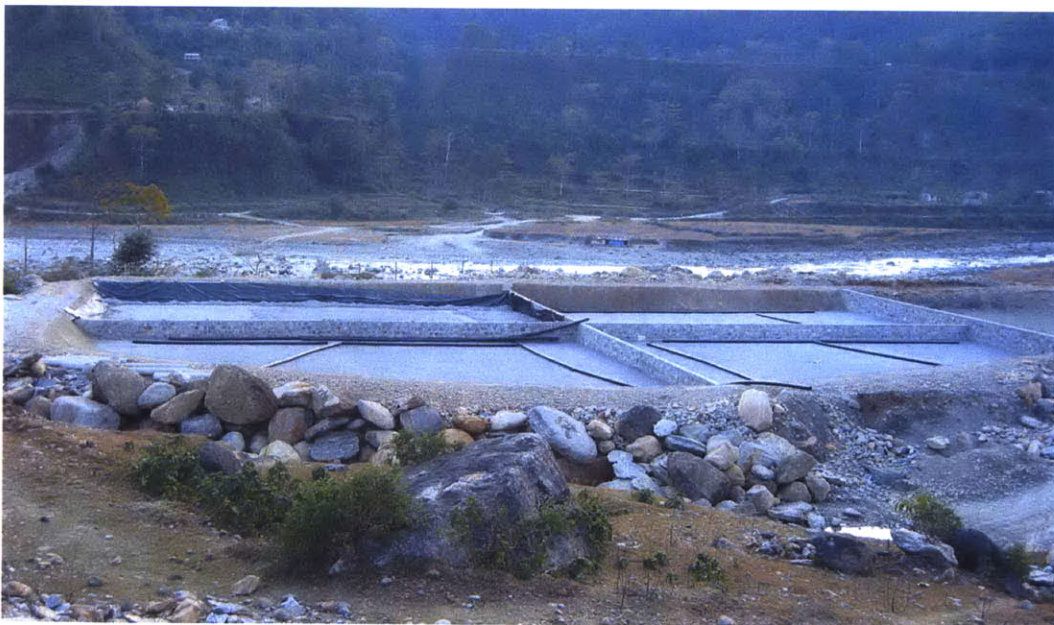
Figure 5.20: Vertical Flow Bed at Kathmandu
