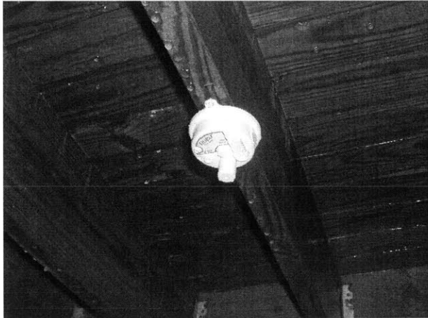
Figure 113f Outdoor temperature sensor located east of building underneath a staircase.
