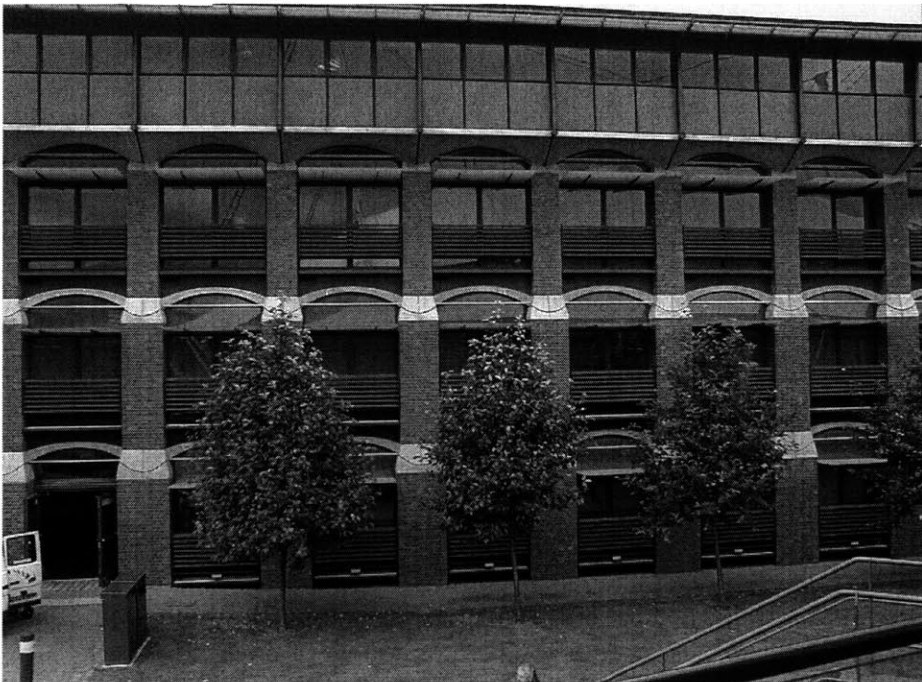
Figure 51 Representative façade. The horizontal bars on the lower three floors are safety railings. Windows open horizontally into the room or can be moved to the side like a typical sliding glass door. Note the external light shields on the third floor. The top floor, featuring a relatively low mass ceiling is reported to be uncomfortably warm during some periods of the summer.
