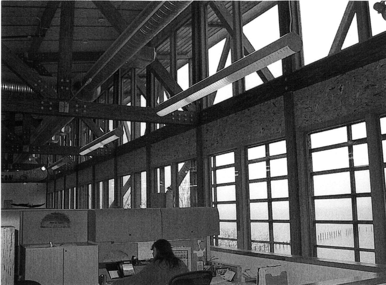
Figure 154 Second floor. All cubicles are fairly low to allow air to pass freely. The solar shading device is clearly visible on the right. The shading device is broken up into two components. For the top bank of windows, a horizontal slatted overhang provides shading, while a vertical wall of wooden slats shades the rest of the windows. Hanging lights adjust to the amount of available ambient light. Sometimes the hanging lights will move when airflow through the building is significant.
