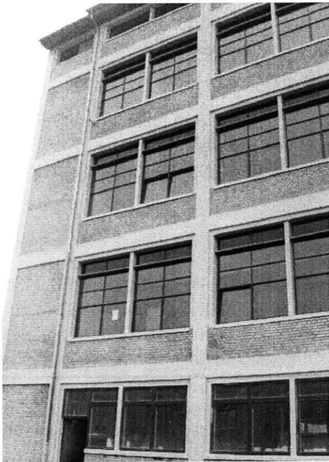
Figure 5 Front façade. Note the tilt windows that are open. The smaller top windows are motorized, while the larger ones are operated manually. The ground floor, which has not been retrofit, is not considered part of the union.
