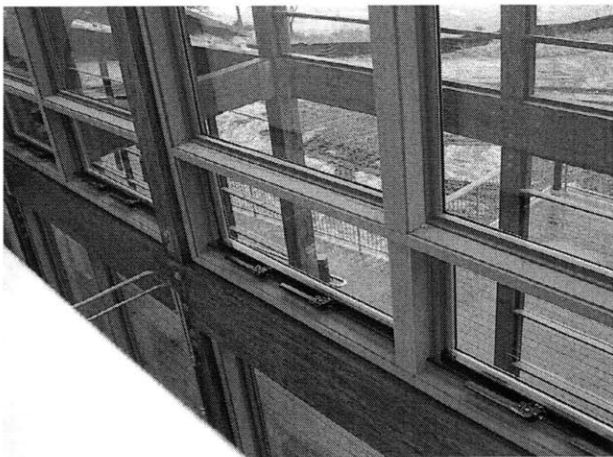
Figure 141 Bank of windows. These windows are located on the south façade. Crank and cable actuators open these top-hinged windows in groups of four.
