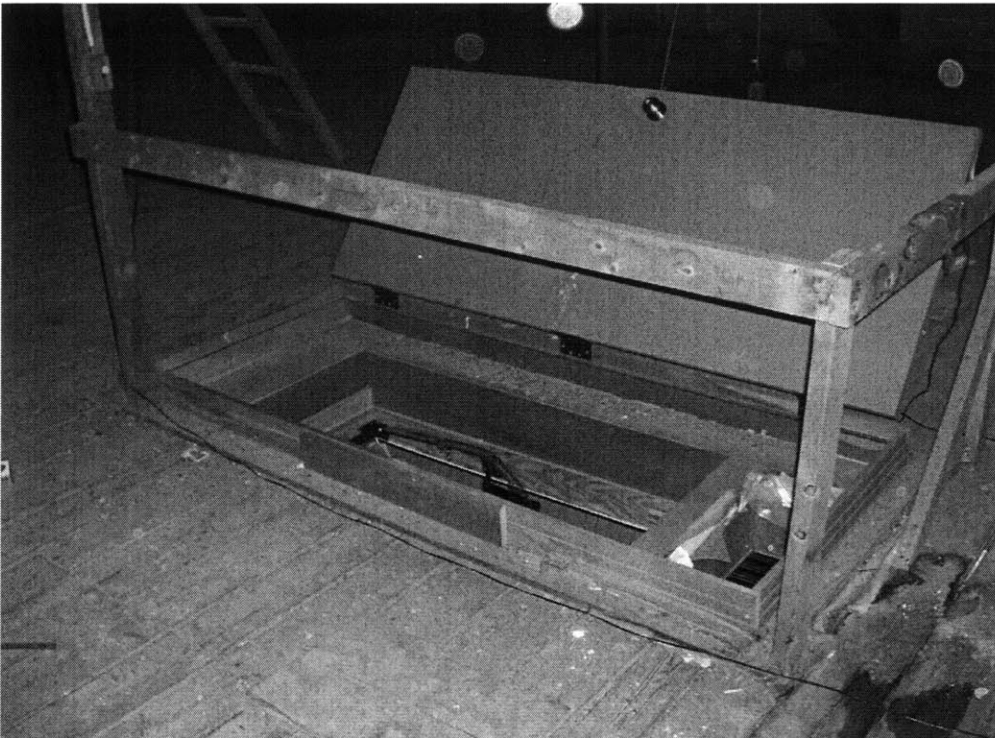
Figure 106 Attic door. This door is closed during the heating season. It is left open at all other times to let warm air to rise into the attic.
