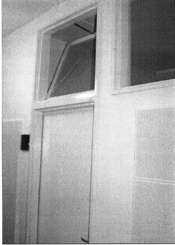
Figure 11 Transom window. These windows allow for airflow movement through interior corridors into three-story atriums. These atriums exhaust air using high-volume fans.
