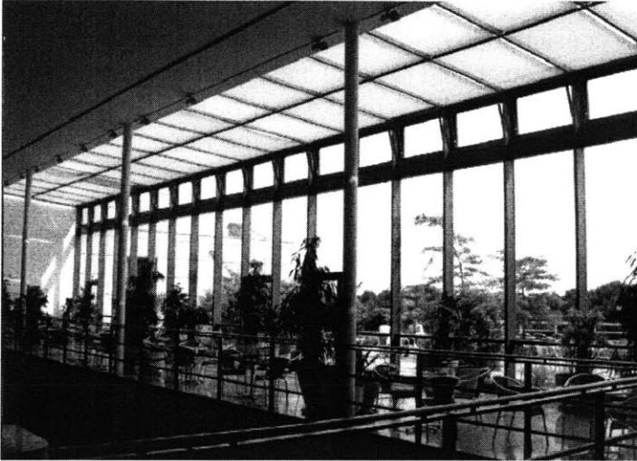
Figure 72 Top-level atrium façade. The windows at the top of the façade are actuated by pistons and opened when stack ventilation is necessary.
