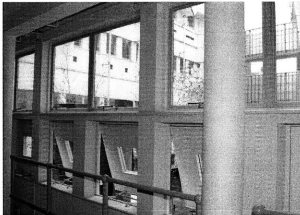
Figure 60 View of typical façade in electrical engineering laboratories. Windows are manually operated.
