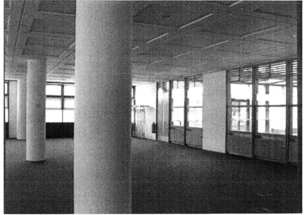
Figure 69 General view of office space. Both the ceiling and the posts are concrete and help with effective night cooling.
