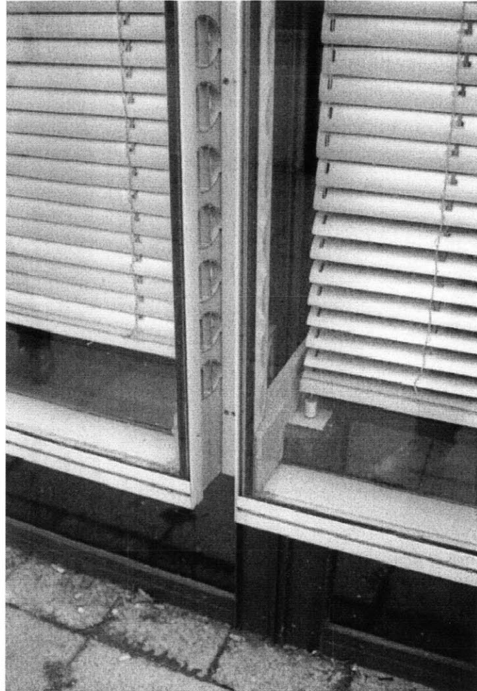
Figure 23 Exterior view of double-skin. Note the V-Channel; the holes are where air enters the double-skin.
