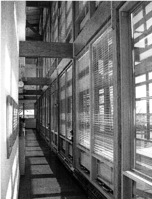
Figure 161 First floor corridor. The rows of windows low to the ground are operable. The open channel allows warm air to rise from the first floor up to the second floor for venting through the clerestory windows. Note the aluminum blinds. They are all operated with cords that reach down to the first floor.
