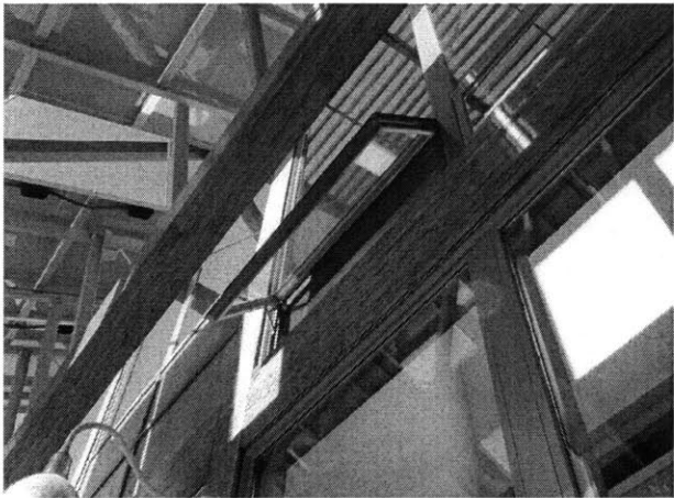
Figure 148 Upper south façade window. In these two window pictures, the crank mechanism was not yet connected.
