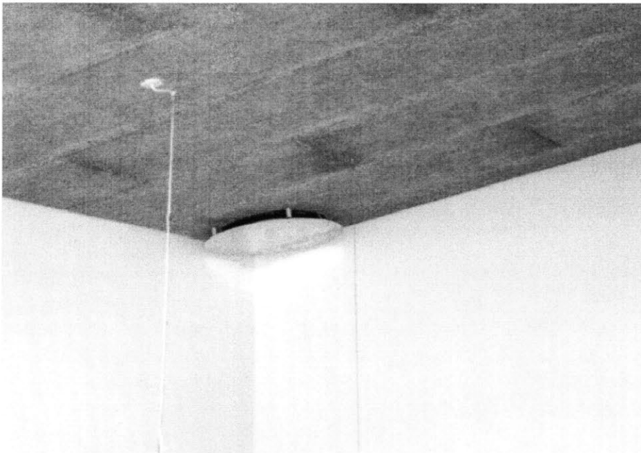
Figure 17 Circular vent in typical classroom. This vent is located at the upper-most portion of a steeply sloped ceiling. The vent feeds into a duct that brings air to one of the ventilation boxes on the roof of the school. It appears that the vent is not configured for optimal airflow. There was likely a trade-off made to make the vent aesthetically pleasing.
