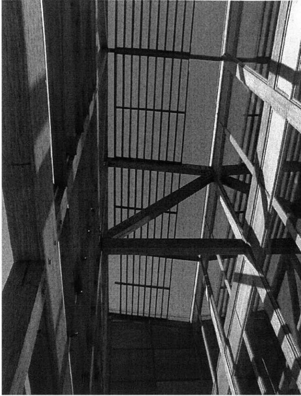
Figure 146 Solar shading device. This device allows low sun to penetrate during the winter, while blocking high sun during the summer.
