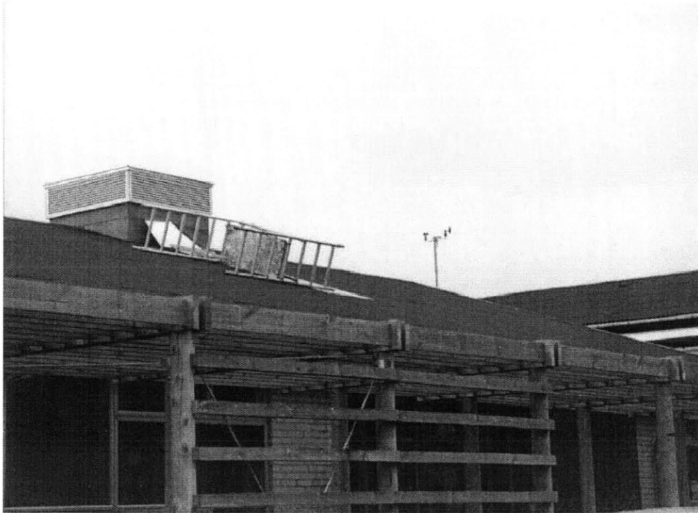
Figure 16 Roof view. Note the ventilation box on the left part of the roof and the weather station on the right. The ventilation shaft exhausts air from vents located in the hallways and in each classroom (see Figure 17). The weather station records wind speed and direction, as well as temperature.
