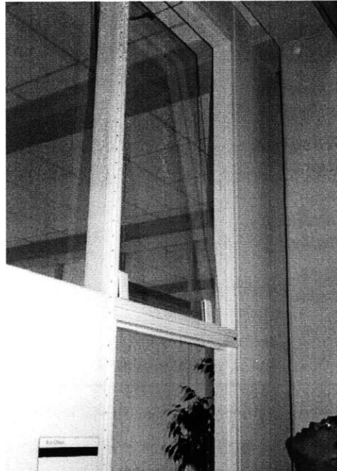
Figure 6 Manually operated transom window. The window allows for cross ventilation through offices and interior corridors. Some objections have been raised over having manual control instead of automatic control for these critical windows. If they are shut, only single-sided ventilation, which is not as effective, is available.
