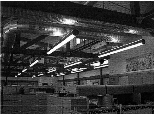
Figure 158 Second floor. Each row of hanging lights can be dimmed in 25% increments. Typically, the row of lights closest to the north-facing back wall, in this picture, is kept on.
