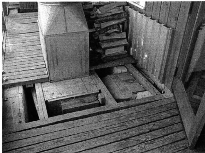
Figure 93 Sunspace fan housing. The fan draws air from the sunspace into the bedrock underneath the concrete basement floor slab.
