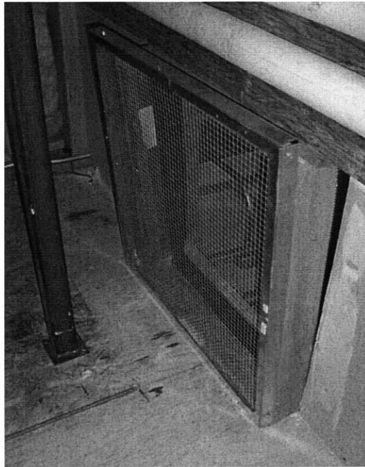
Figure 162 Air vent. This vent is located in the mechanical room on the second floor. When the natural ventilation fan in the mechanical room is operating, air is brought from the occupied spaces through this vent.
