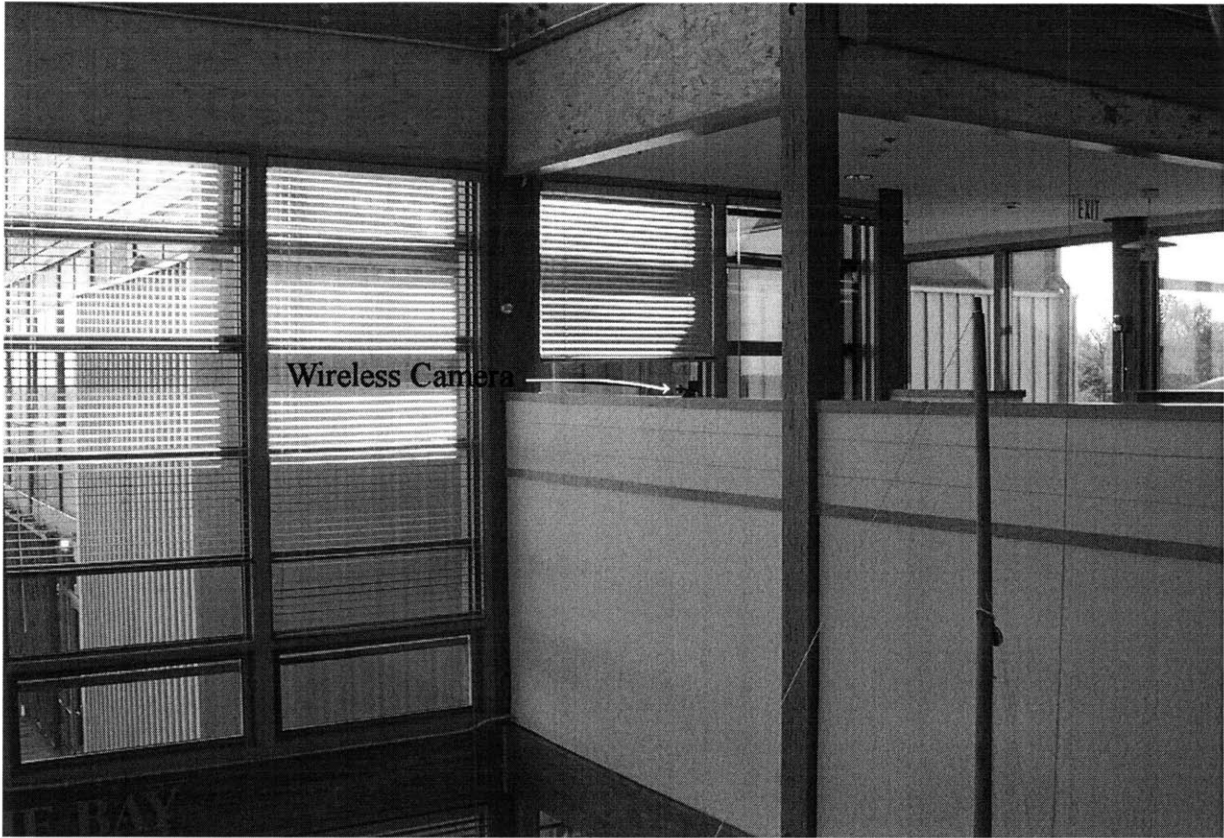
Figure 163 Wireless camera. The camera sits unobtrusively on a ledge to view the status of windows on the south façade.
