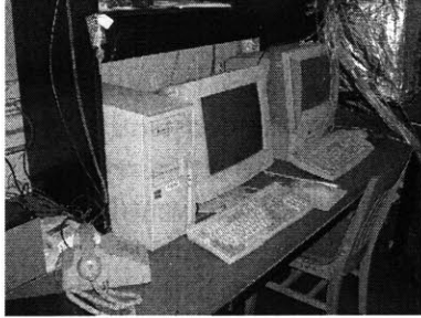
Figure 116a Tracer gas computer controller.
