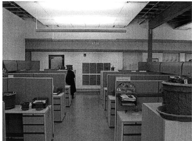
Figure 153 First floor east office area. The large vent on the rear wall feeds to the larger of two natural ventilation assist fans.
