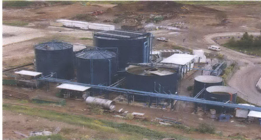
Figure 17: Two-phases anaerobic digester. 142
