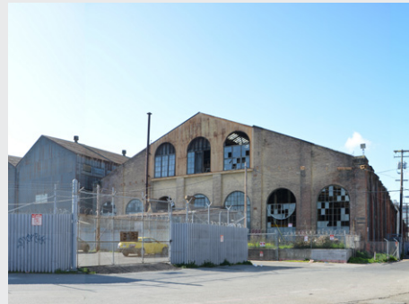
Building 113/114: Union Iron Works Machine Shop “Very Significant Resource” to be rehabilitated by Orton. 90,000 sf; steel and brick; built 1885
