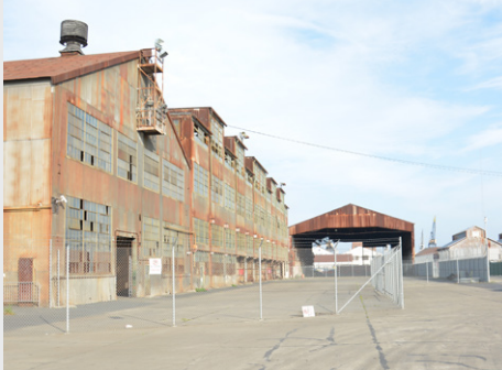
Building 12: Plate Shop No. 2 “Significant Resource” to be rehabilitated by Forest City. 118,890 sf; steel frame/wood floor; built 1941
