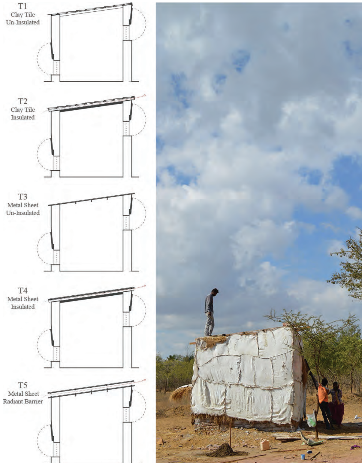
Figure 5.1 – Left: Five test chamber types for reference. Right: Chamber construction at Paraspar.
