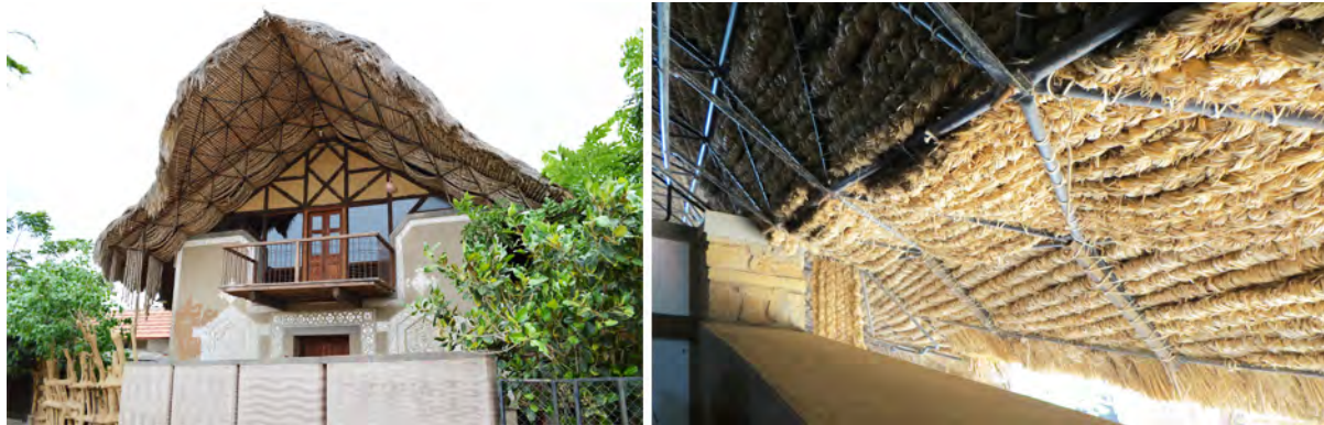
Figure 3.10 – Exterior images of Building 5. Left: View of the southwest facade. Right: Interior view of thatch roof overhang and open-air clerestory window.
