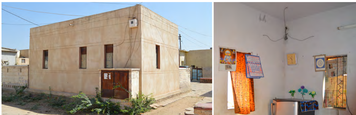
Figure 3.22 – Images of Building 7. Left: View of the southwest facade. Right: Interior view of the uninsulated CSEB walls and RCC slab roof.
