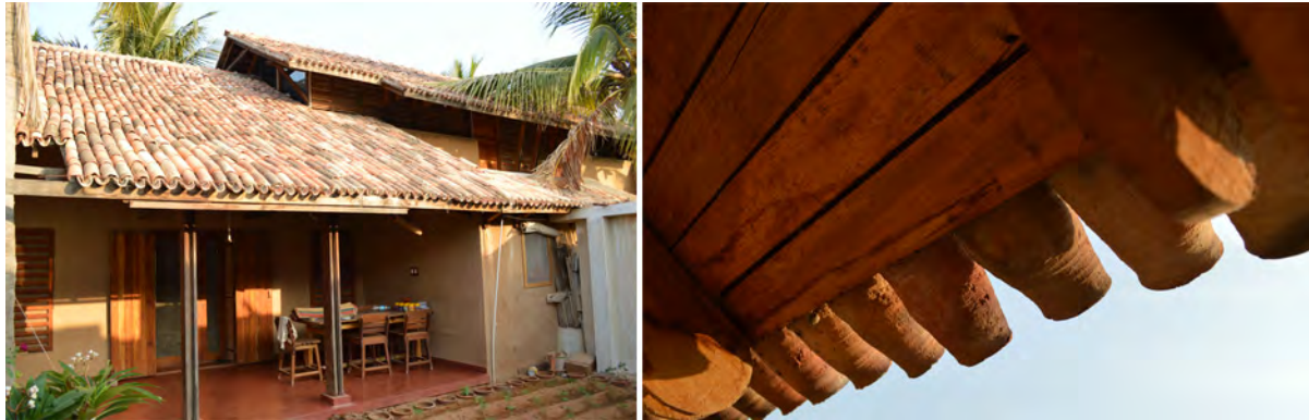
Figure 3.4 – Exterior images of Building 2. Left: Looking at a portion of the building from the west. Right: close view of exterior roof country tile detail.
