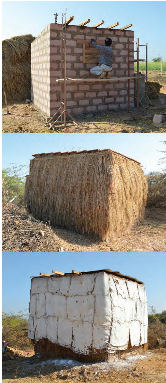
Figure 5.4 – Test Chambers in Various Stages of Construction. Chamber walls are constructed from 23 cm local sandstone block (top) and then insulated on the exterior with straw thatch panels (middle). Walls are further protected from the sun and outdoors with an outer finishing of burlap sacks coated with lime plaster (bottom).
