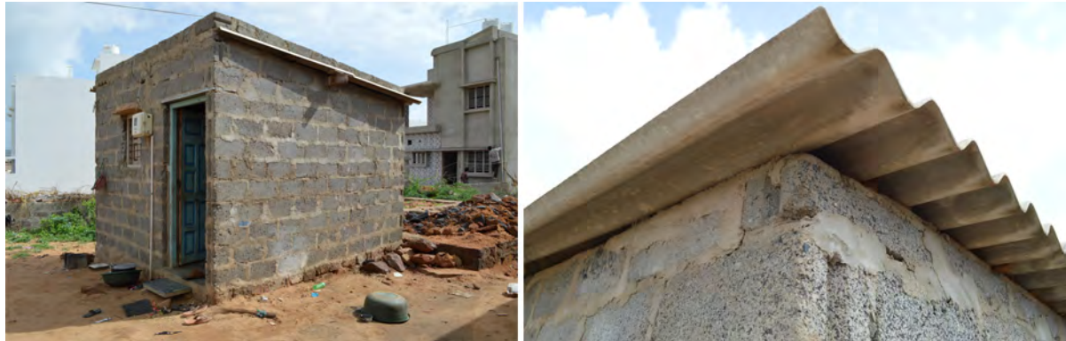
Figure 3.2 – Exterior images of Building 1. Left: Looking at the building from the northeast. Right: close view of exterior roof to wall connection on the southwest wall.
