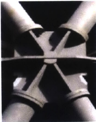
(a) Steel HSS Node
