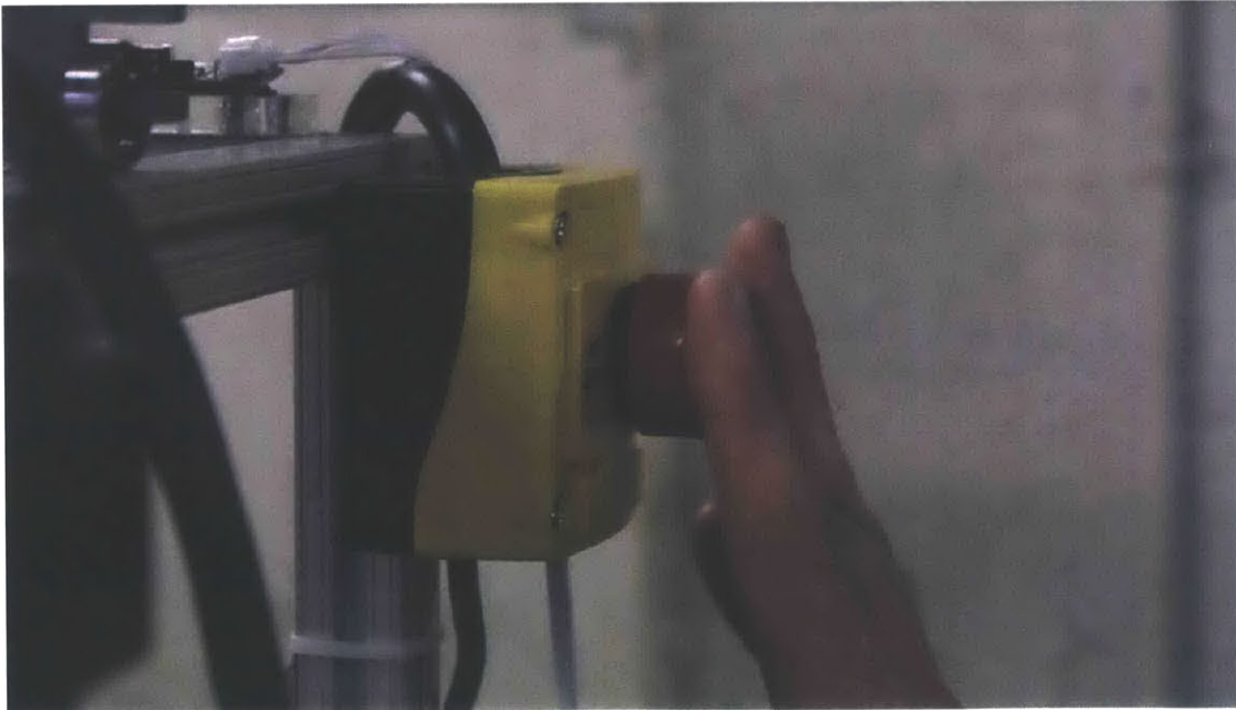
Figure 22: Emergency stop button
