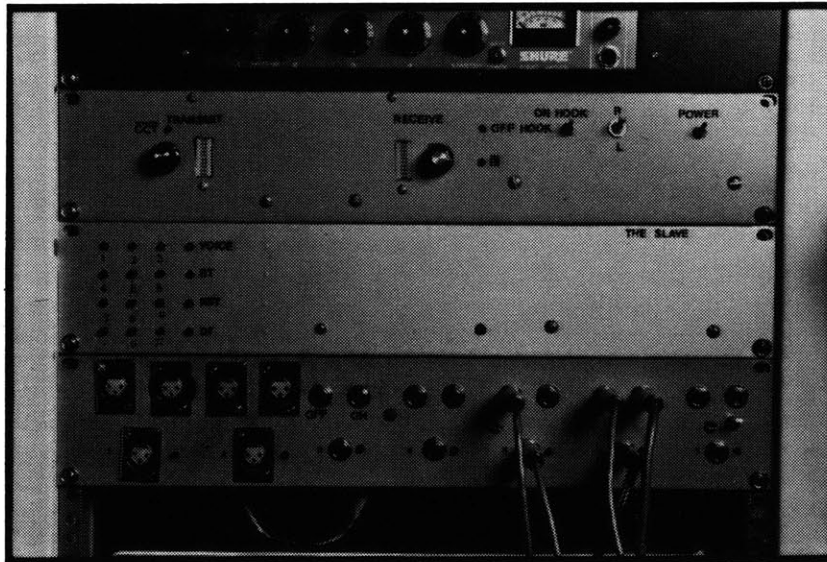
The phonebox: 2-4 wire converter, DTMF decoder, and audio switches.
