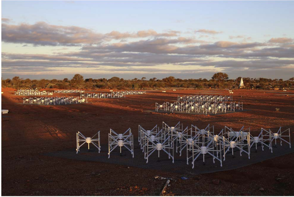
Figure 1. MWA Phase II tiles in the Murchison Radio-astronomy Observatory in Western Australia. (Taken by Greg Rowbotham in 2016 June, when Phase II was under construction.)
