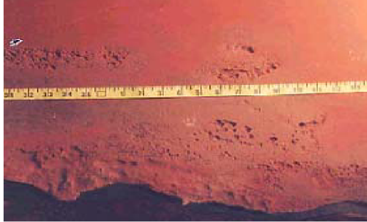
Figure 1-4: Pitting Corrosion [Baker, 2008]
