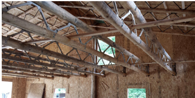
Figure 21: Trusses with whole timber chords and steel web members are used as spanning elements in the Hanifl garage project. (Gundersen, 2015, WholeTrees, n.d.b). Photograph courtesy of WholeTrees Structures.
