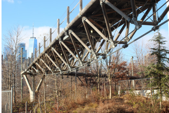
Figure 20: Naturally durable round Black Locust timbers are used in an underslung cable arrangement in the Squibb Park pedestrian bridge (Woodward and Zoli, 2013).
