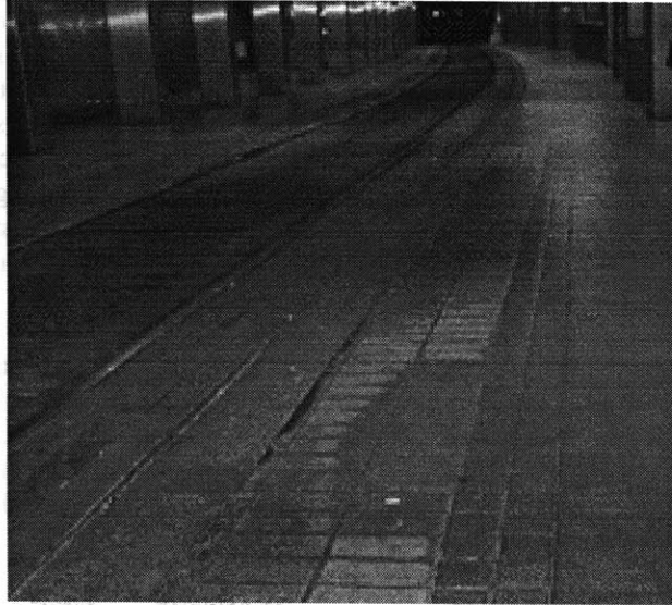
FIGURE 5. Wear in the station (floor closeup)
