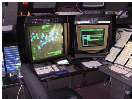
Figure 3-12: The primary means of control for the New York and Oakland Center controllers is paper flight strips ( right ). A situation display is also available for reference ( left ).
