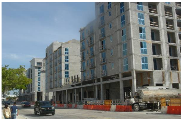
The new Downtown Kendall under construction Mixed-use buildings with underground parking shown Source: Amy Merritt
