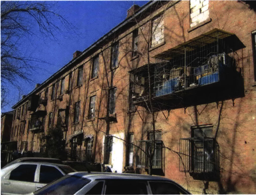
Photo 5 Typical existing residential buildings in Jing Mian communities, which were built in the 1950s.
