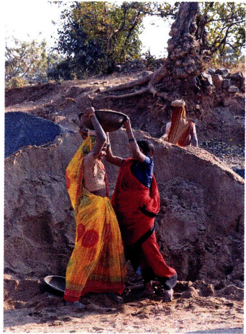
IN A PERPETUATION OF PATRIARCHAL CONTROL INTO LABOUR SYSTEMS - WOMEN OCCUPY THE BOTTOM RUNG OF THE LABOURERS ON AN INDIAN CONSTRUCTION SITE, LIFTING THE HEAVIEST LOADS WHILE MALE WORKERS CARRY OUT MORE SKILLED TASKS.
