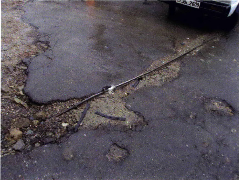
Figure 7: A Leaking Pipe with Plastic Taping
