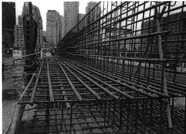
Figure 2.23: Reinforcement cage for a T-Slurry wall, (MBTA Courthouse Subway Station, South Boston)
