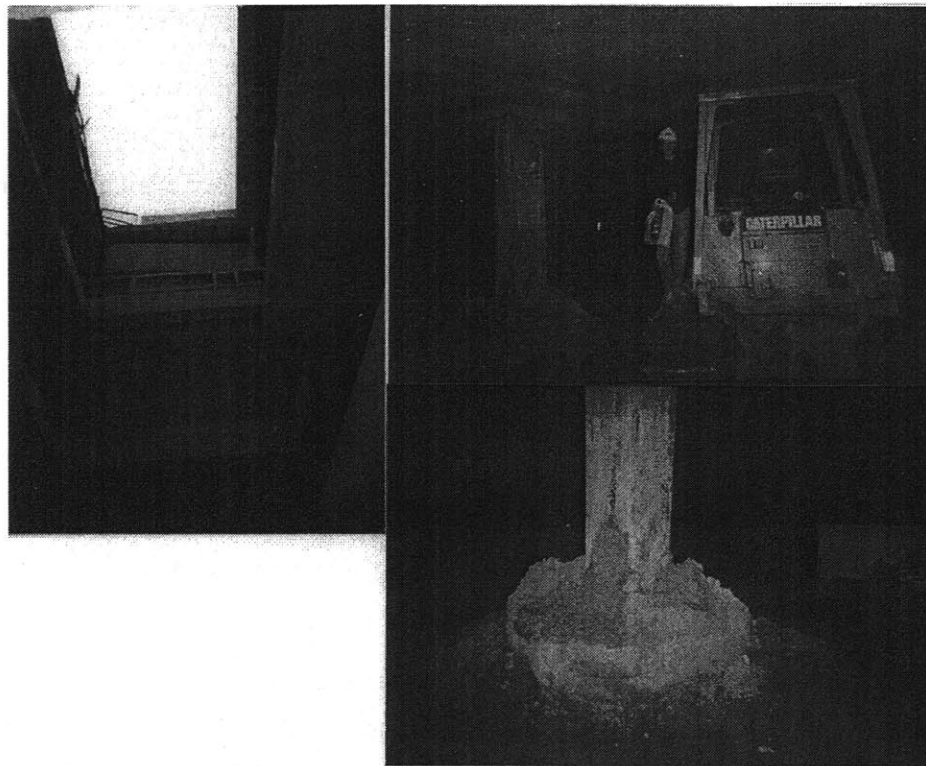
Figure 2.33: Millenium Place excavation. Left: Looking up at a glory hole, Top right: author in the lowest most level note LBE on the left and the barrette, Bottom right: close up view the same barrette (LBE) and steel beam (B13).
