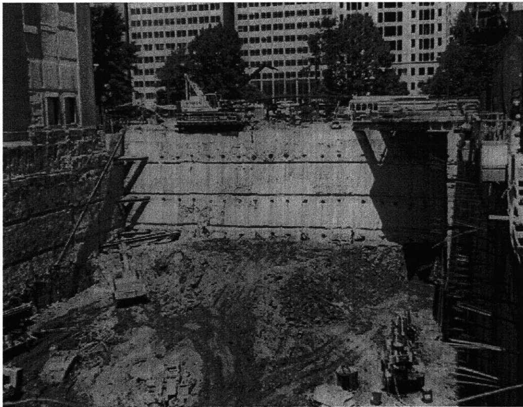
Figure 2.24: Picture from a tieback slurry wall excavation (World Bank Project Washington, Case Study W-1)
