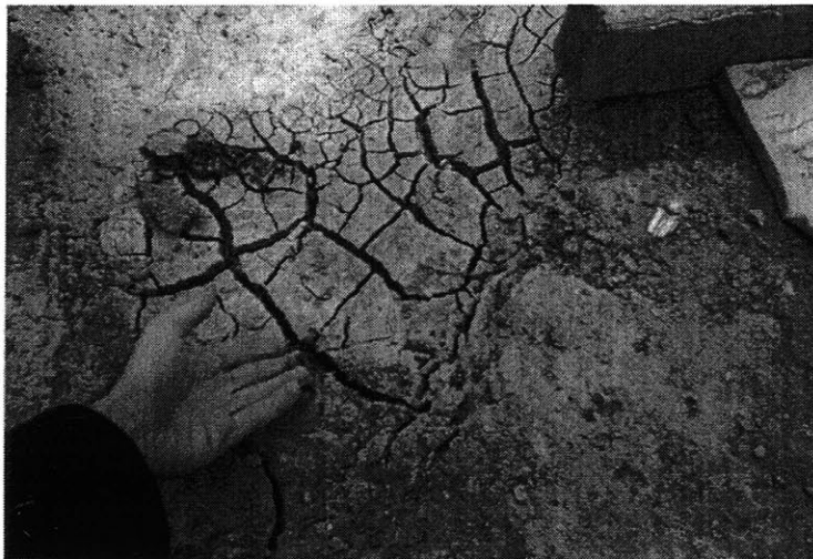
Figure 2.16: Top concrete layer, slurry contaminated concrete easily crumbles with finger pressure (author's hand), note fissures at the concrete
