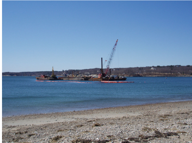
FIGURE 1. Barge and dredge located over eelgrass bed at Pavilion Beach during outfall construction.
