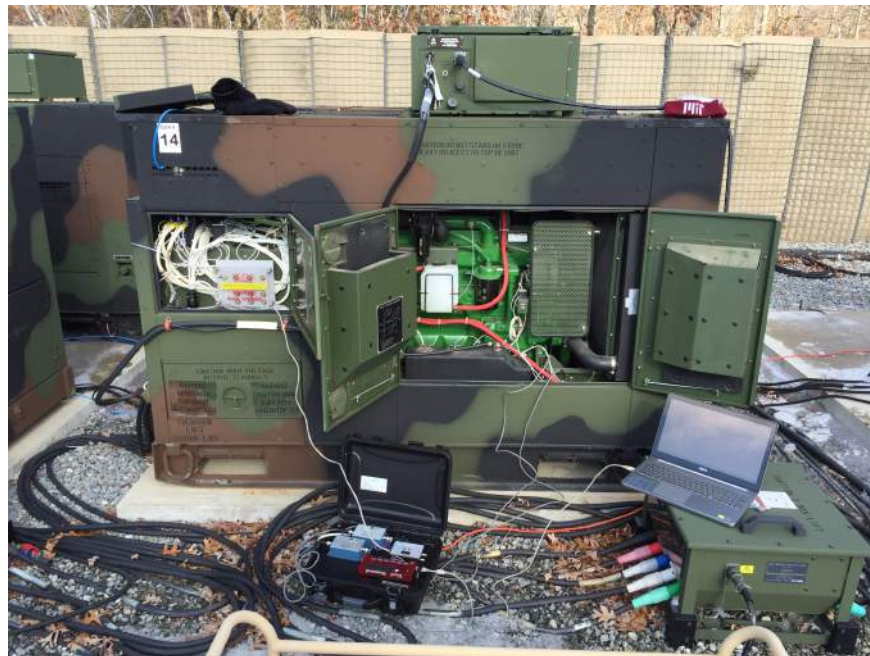
Figure 3-21: Fully Instrumented Generator at Fort Devens
