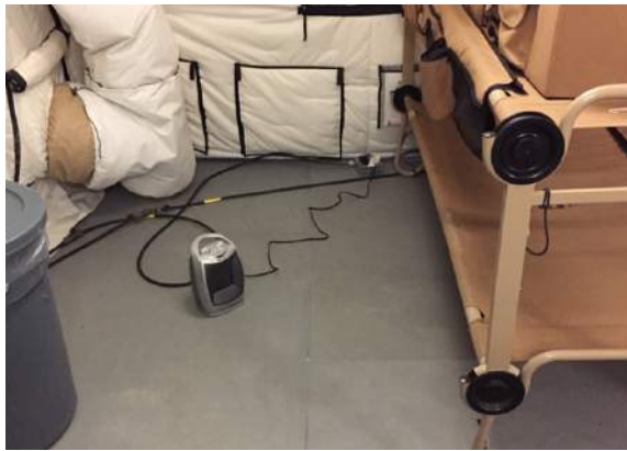
(b) Space Heater in Tent Corner
