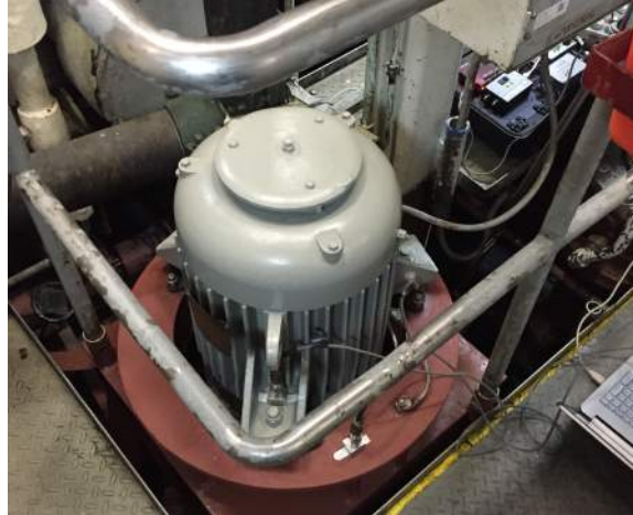
Figure 3-30: MCM ASW Pump
