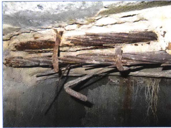
Figure 8: Corrosion of pre-stressing tendons within Hammersmith Flyover, London [12]
