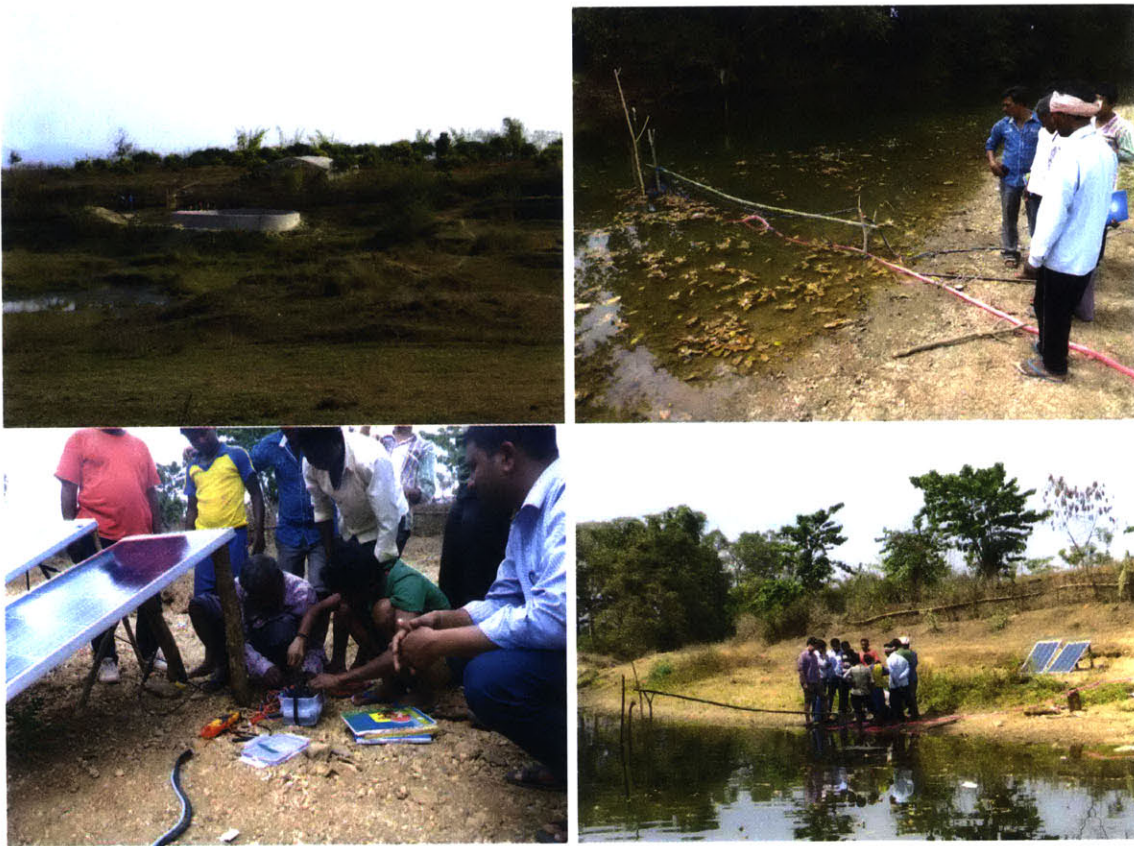
Figure 4-10: An image of the water source below the fields (Top Left). The pump secured to a bamboo structure in a river at the second site (Top Right). Training for operation and maintenance of the electrical system (Bottom Left). Training for proper installation of the pump (Bottom Right).
