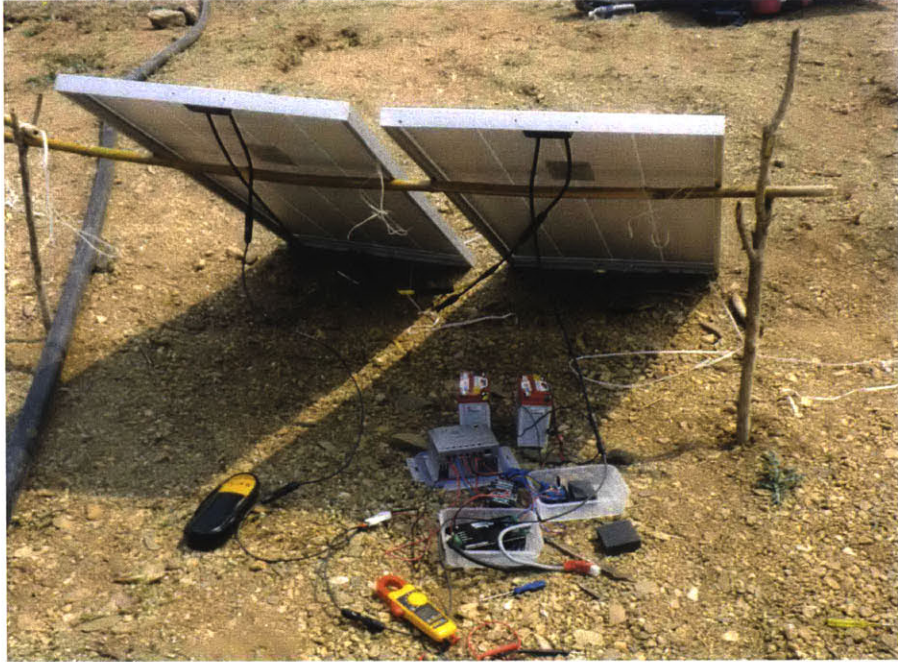
Figure 4-5: Panels, charge controller, motor controller, Arduino Uno, and batteries wired up for use along with some tools for debugging.
