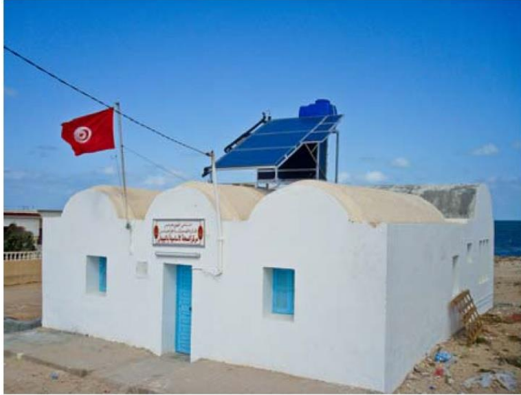
Fig. 1-1. Solar-powered Oryx 150 membrane distillation system installed in Tunisia [5].
