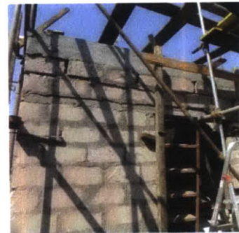
Separation Cracks Above The Lintel Level
