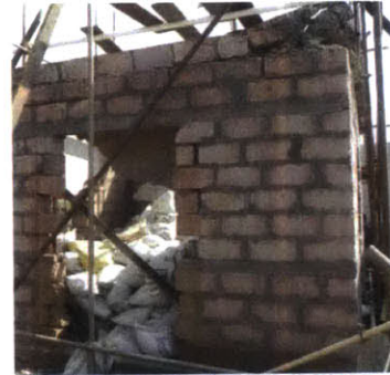
Structure After The Loading Test
