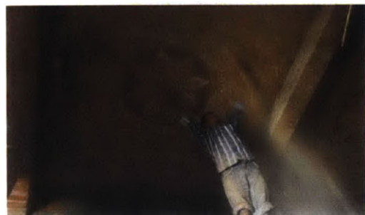
AFTER THE SHUTTERING IS REMOVED, THE DOME IS CLEANED AND ANY SOIL IS SCRAPED OFF.
