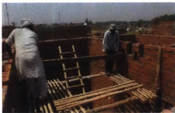
1 MS 1 SECTIONS (GIRDERS) ARE PLACED INTO THE GROOVES MADE IN THE WALL
