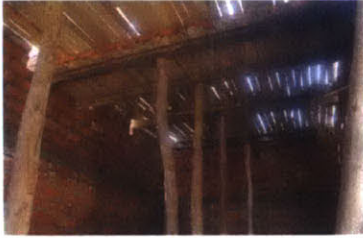
SHUTTERING IS DONE. PLANKS ARE PLACED ON THE SAME LEVEL OF THE BEAM
