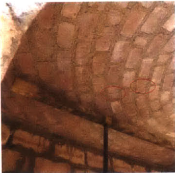
Cracks Appearing Near The Corners
