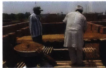
2 WOODEN PLANKS ARE PLACED ON THE GIRDERS, SANDY SILTY SOIL IS LAID ON THE PLANKS.
