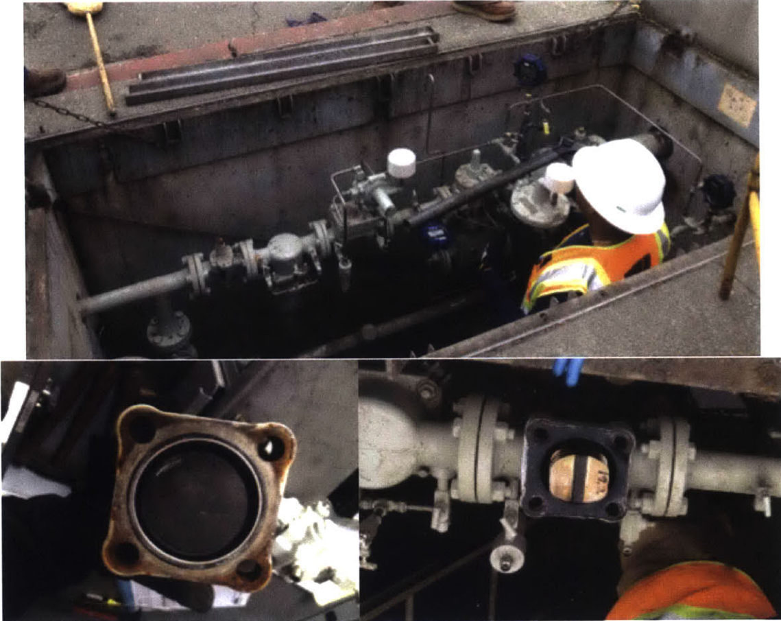
Figure 1-2: Distribution regulator undergoing maintenance
