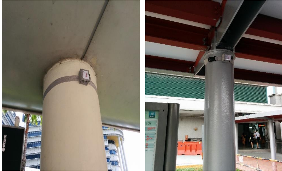
Figure 6.4 - Beacons installed at bus stops
