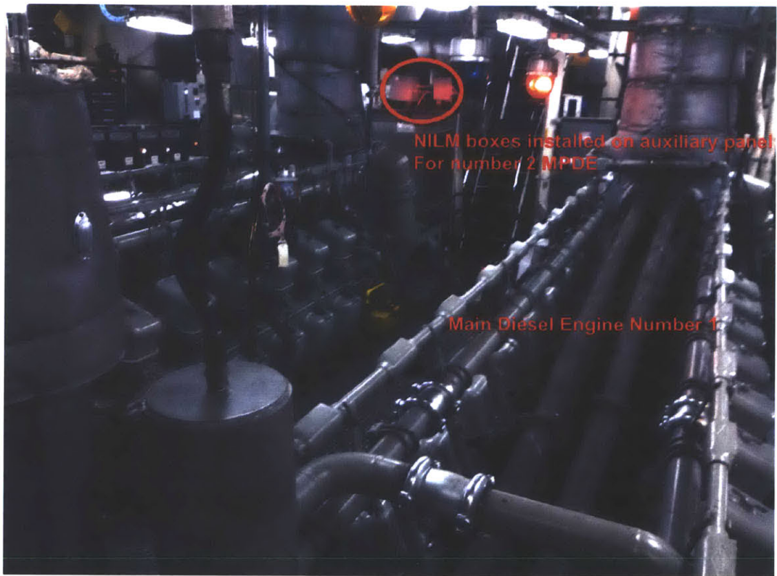
Figure 5-18: USCGC SPENCER engine room. Nonintrusive monitors are installed forward of the #2 MPDE just above the monitored panel.
