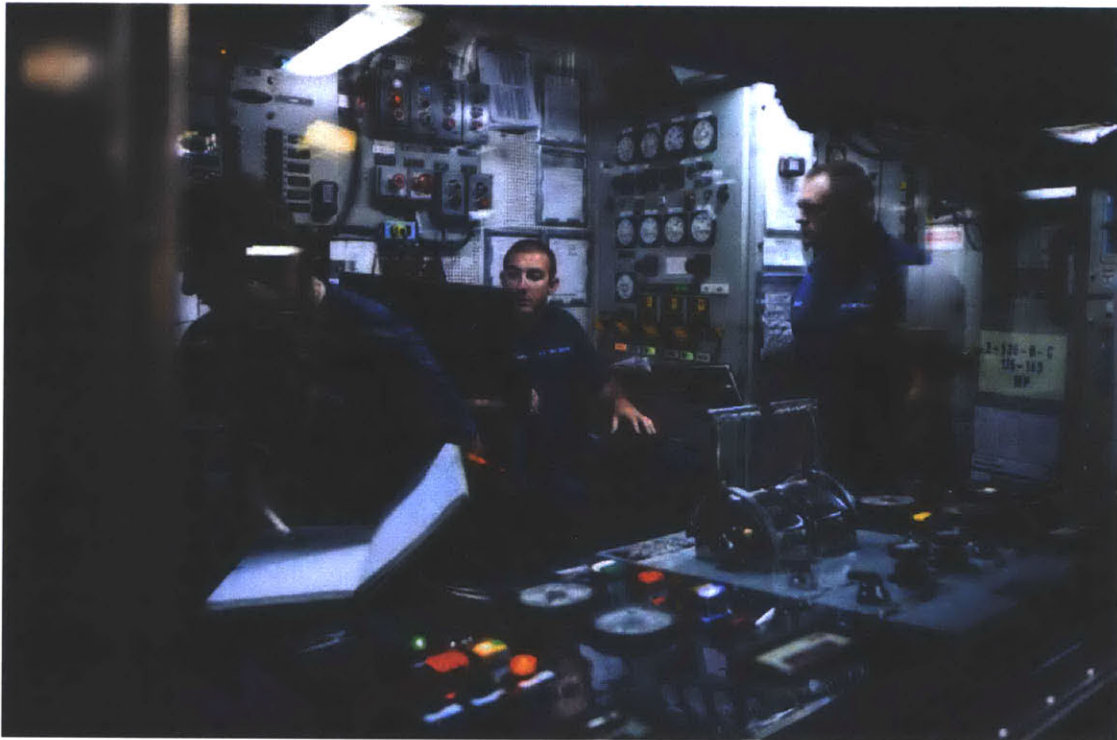
Figure 5-15: Typical USCG engine room watch. Notice the logbook, termed the “rough log,” used to keep machinery operation times and log critical events. Also note the watchstanders monitoring equipment while simultaneously attempting to maintain logs.
