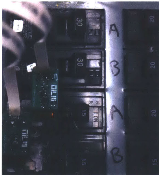
Figure 3-2: Monitoring a circuit breaker panel with TMR sensors
