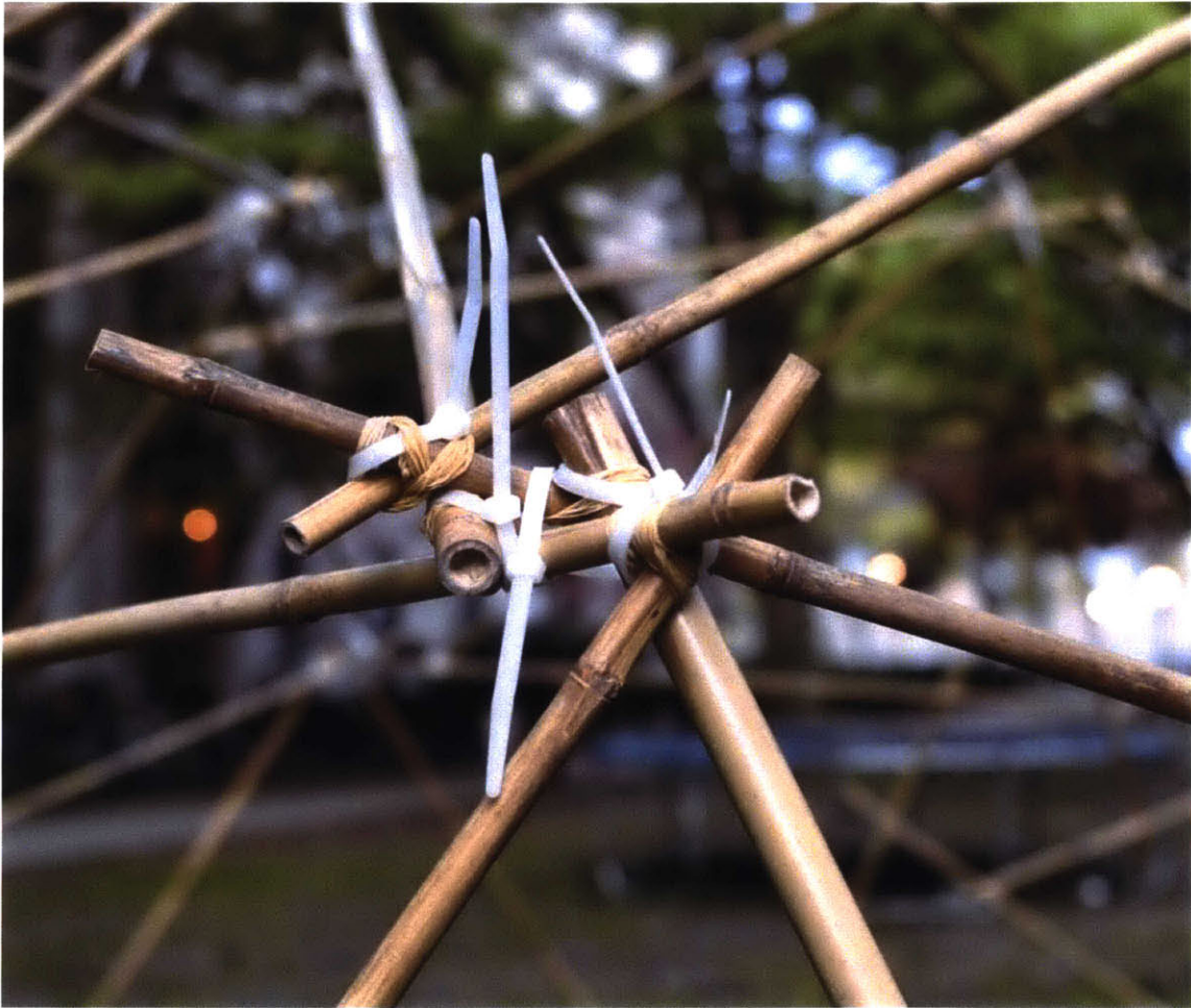
Figure 4-21: Photograph to show some of the messy joinery.
