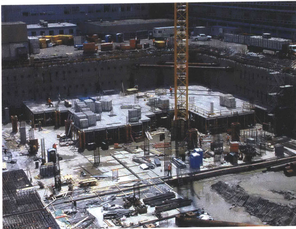
FIGURE C-31: Construction of the slab for the second floor starting in the Southwest corner.
