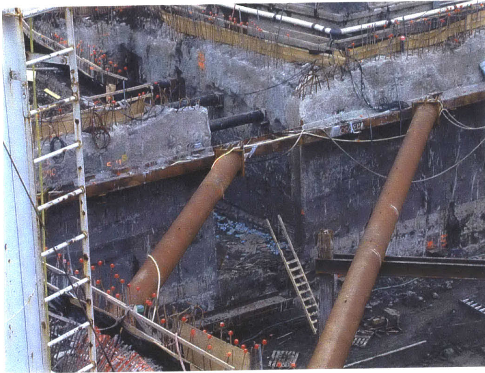
FIGURE C-24: Slurry wall opening in the SE corner for exhaust structure, and wale used to bridge the opening.
