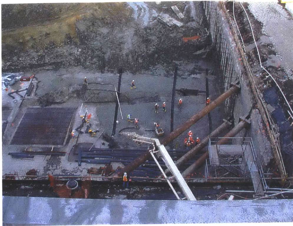
FIGURE C-30: Placement of strip drains below the mudmat, and construction of the mudmat.
