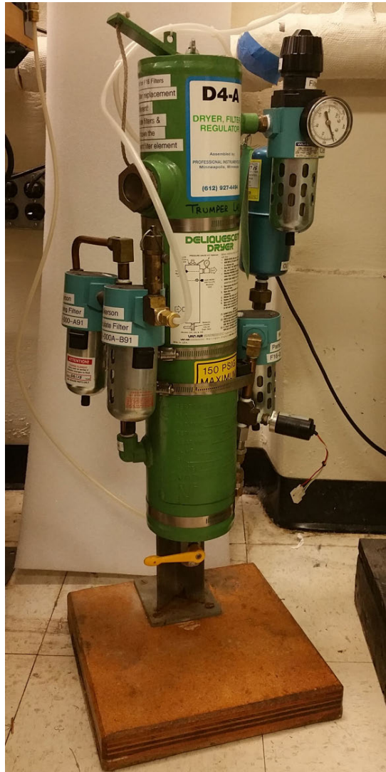
(b) Stage 2: Chemical air dryer with progressive filtering to remove oil from the air.
