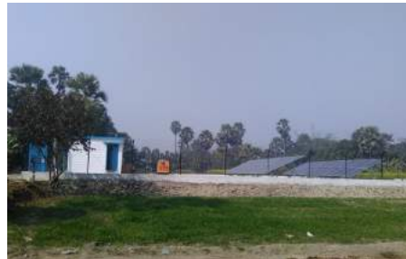
(c) Side view of the microgrid's battery and control system housing, diesel generator, and solar panels
