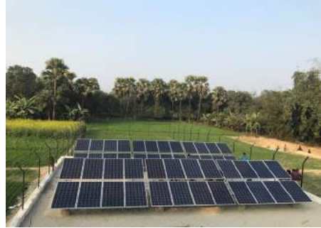
(b) Aerial view of the microgrid's solar panels
