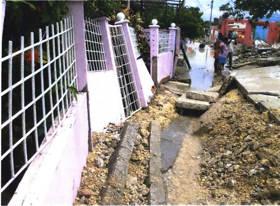
Image 14: Impacts of floods in SF
