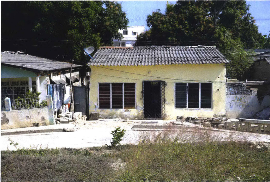
Image 1: Original design of the house from the Territorial Credit Institute in SF
