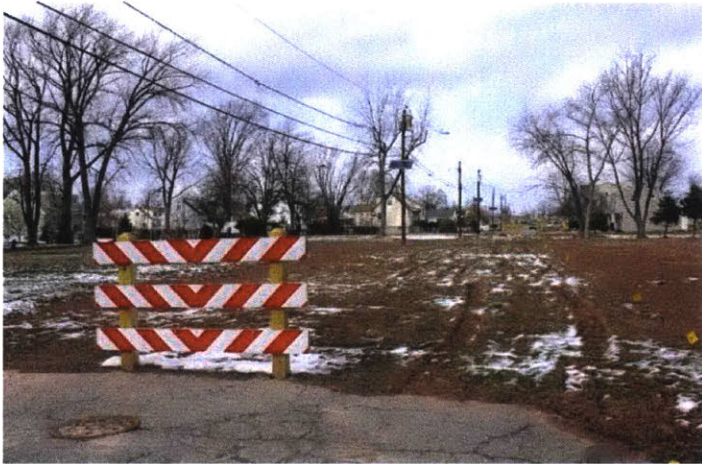
Figure 5.8: A stretch of Watson Road has been recently removed while the powerlines are, at least for now, still in place. Woodbridge, NJ. Photo by Author
